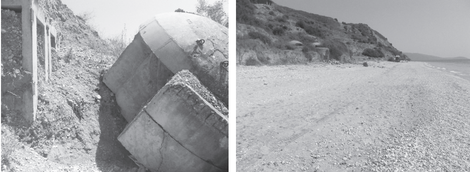
Figure 7. Two cases of bunkers state in southern area of the beach, left (a) a crushed bunker as result of basement (road track) erosion and (b) two bunkers still in their original position but with a partially eroded basement. The case (a) is located in the half of distance from coastline compared to case (b). In the picture on right (case b) can clearly observed the setting of beach sediments from earth toward coastline in ranking gravel-sand-gravel. The sandy layer is separated from the sea by actual berm of coastline (Image S. Marku 2015).
