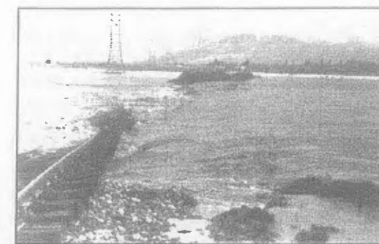
Photo 1- Photograph looking to North (10 km in north of Lezha town). A damaged railway (Lezha-Shkodra line) caused by flooding of 1998 year.
