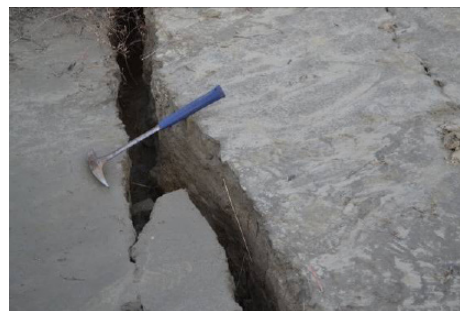
Figure 8. Cracks in Juba created during the earthquake of No-venber 26, 2019
